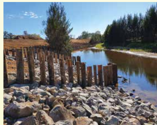
Completed work at the first location include earthworks to batter the site, installation of pile fields and revegetation.
